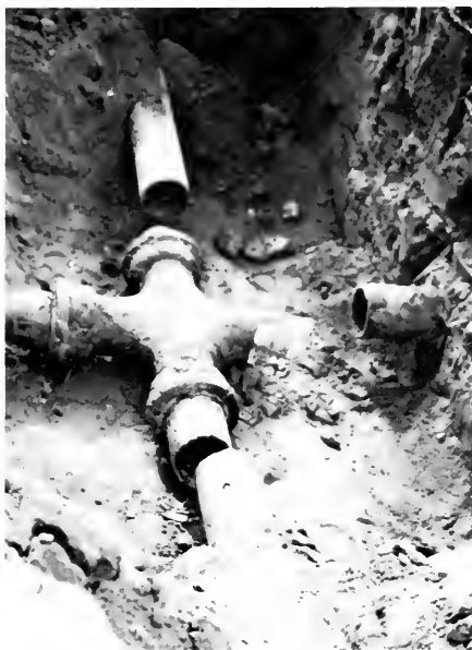
Photo 50. Typical view of water pipe joint separations and shears near joints.
